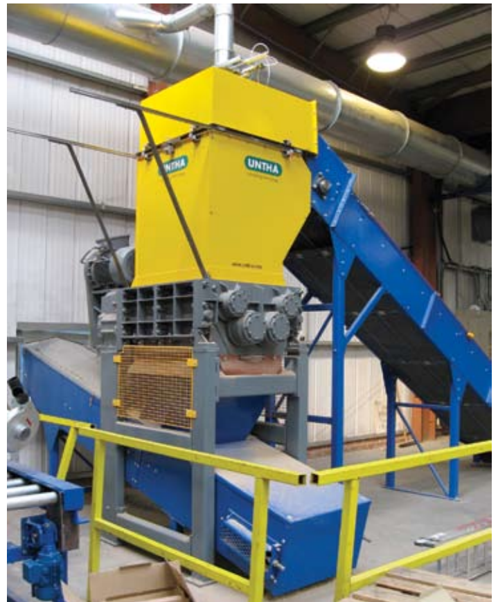
The Kingspan recycling shredder at the company's Hull site.
